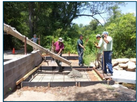
Interns and staff at FWNCR pour concrete for an access ramp for a floating dock.
