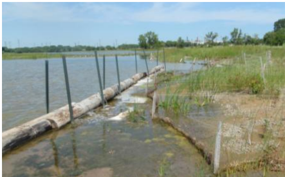
Log structure to protect newly created sand island from wind and wave erosion
